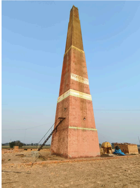
Non-Operational Bhatti, Ladder, Gravitational Settling platform
